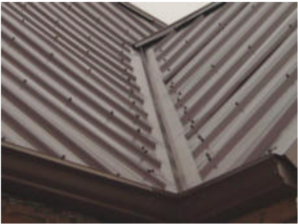
Not allowed - fasteners are exposed
